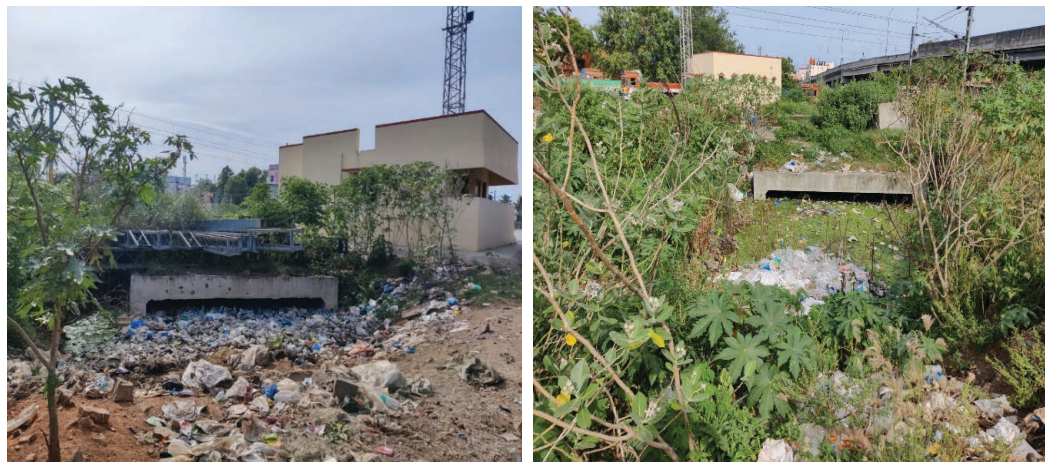
Abandoned LUS Work between Tirumani and Chengalpattu
