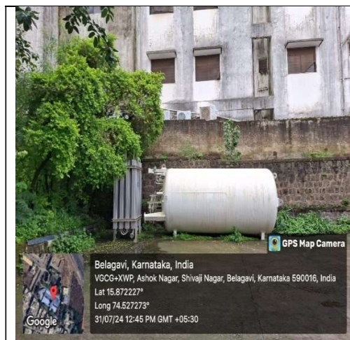
Exhibit 15: Liquid Oxygen Generator lying idle in open yard of ESI Hospital, Belagavi
