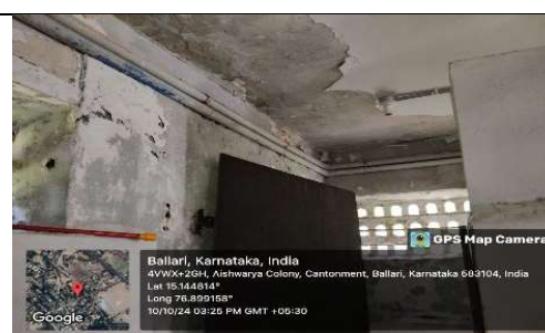
Exhibit 10: Cracks and water seepage in Ballari hostel
